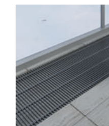
Fancoiled Heating behind a grill
